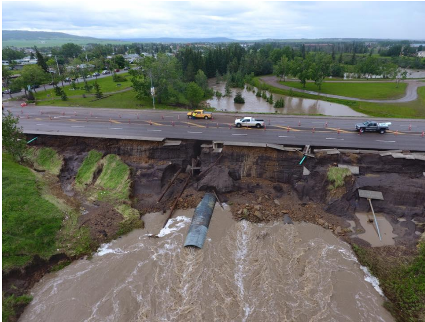
Figure 9: 8th Street in Dawson Creek following flood event - June 2016
