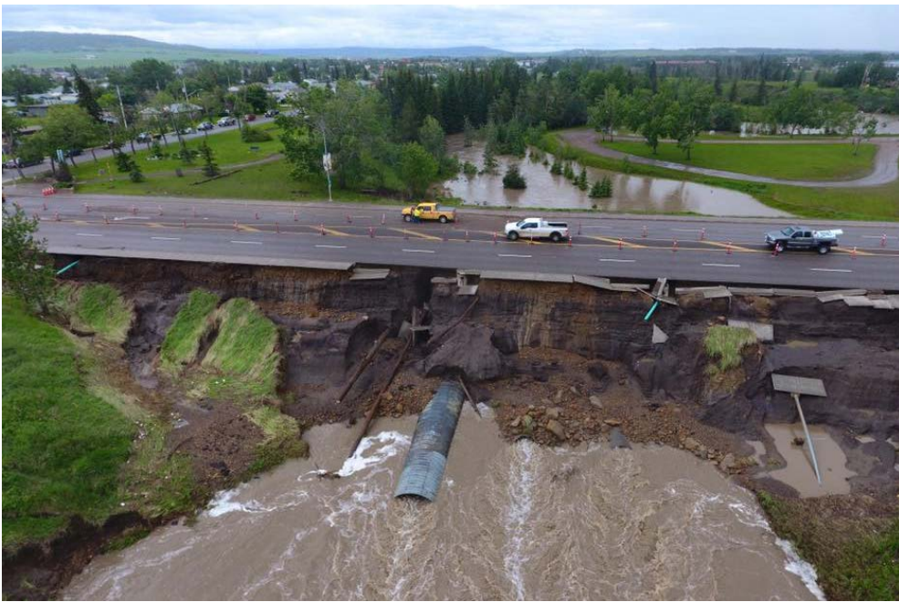
Figure 4: Aerial photo of damage to 8th avenue in Dawson Creek due to 2016 flood looking upstream (west) 4
