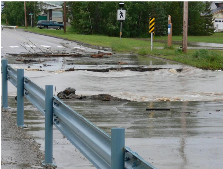
Figure 8: Flooded 15th Street Crossing - Dawson Creek June 2016
