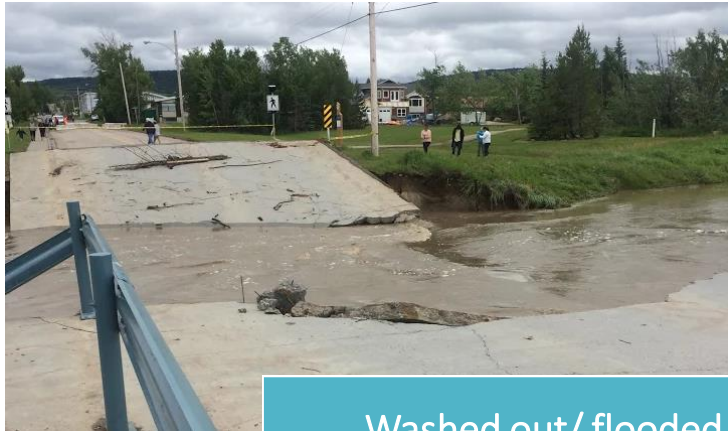
Washed out/ flooded roads
